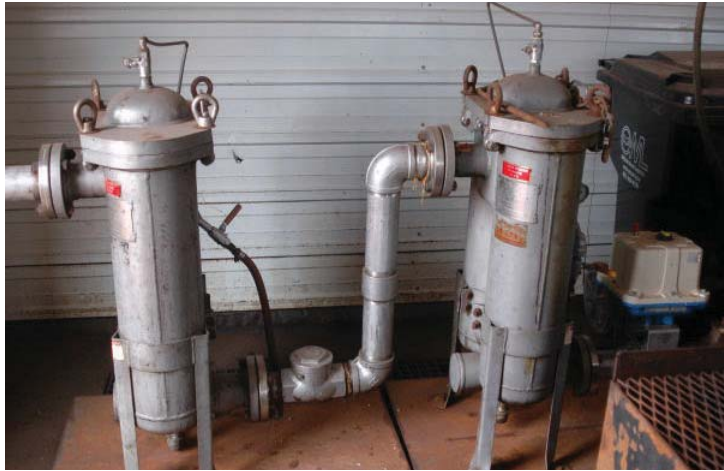
Injection well paper filter containers
